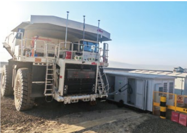
The first set of 1.5MW skid-mounted 4-gun liquid-cooled charging project in China [Huolin Gol,]
