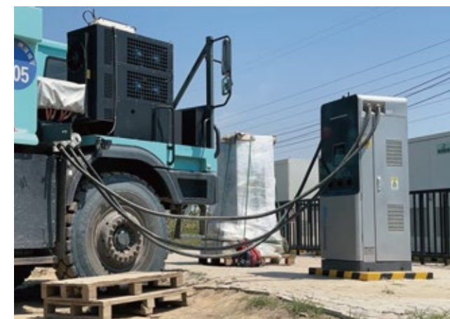
▲ In 2022, the first 1.8MW 3 guns liquid-cooled charging project in China [Ordos, Inner Mongolia]
