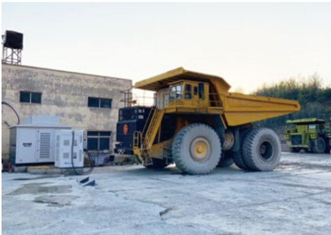
The first set of single-gun 1500V 1500A mining truck charging project in China [Anshan, Liaoning]
